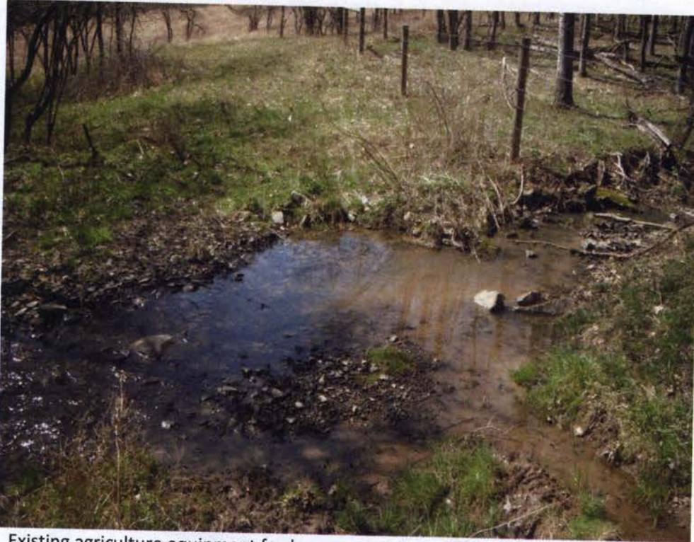
Existing agriculture equipment ford access crossing in the southern half of the site.
