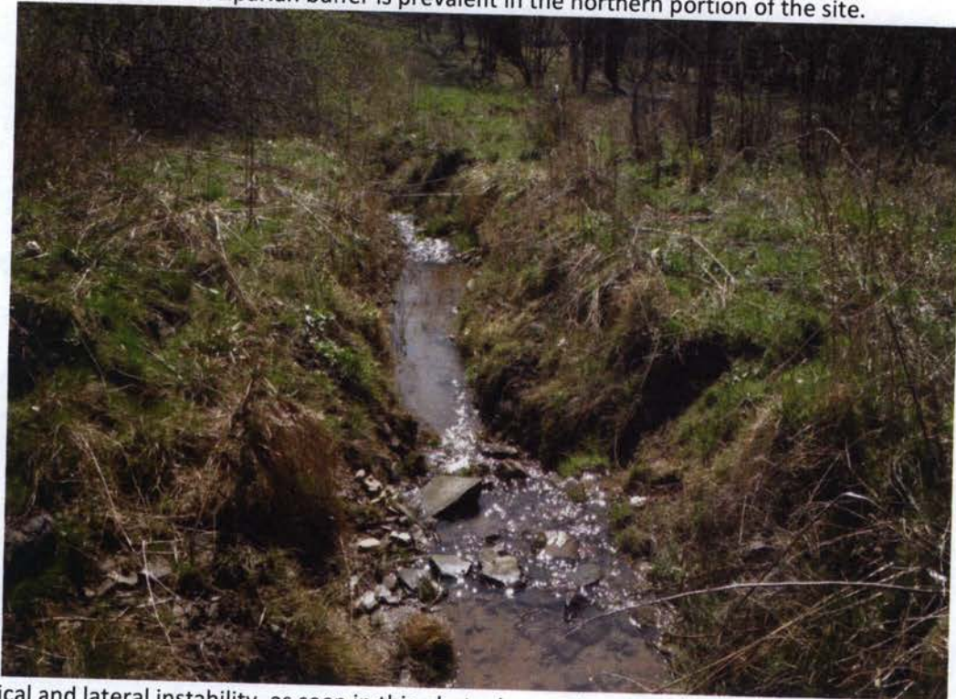
Vertical and lateral instability, as seen in this photo, is prominent within the northern portion of the project site.
