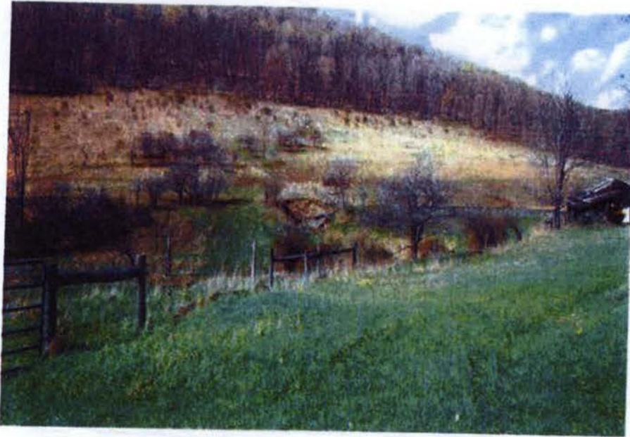
Photo 19 (Facing Northwest – March 2012) – Overview of pond and vicinity including earthen berm, failing outfall, and deteriorating outbuilding.
