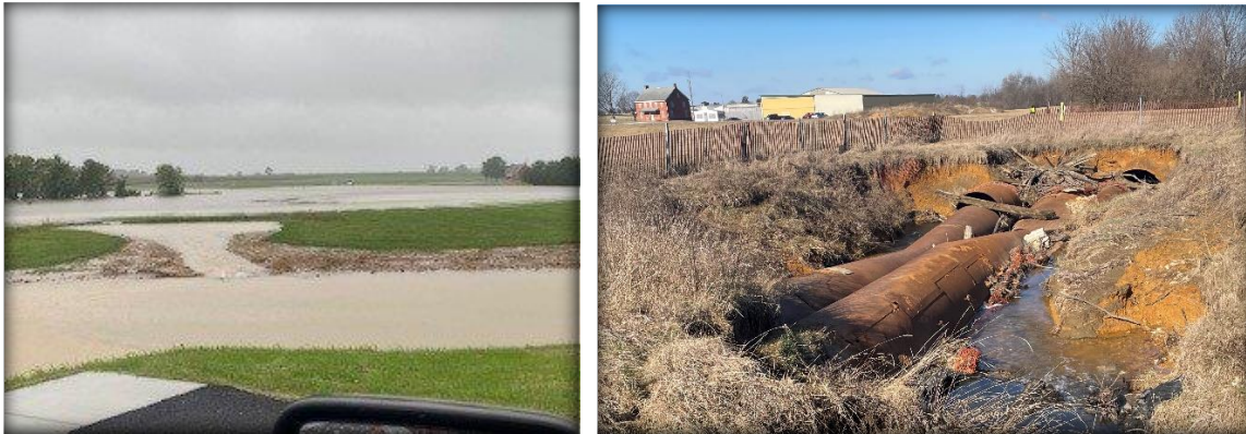
Figure 3, Left picture showing the lake effect from the blockage, right picture showing the sinkhole and tangled culverts causing the backwater.
