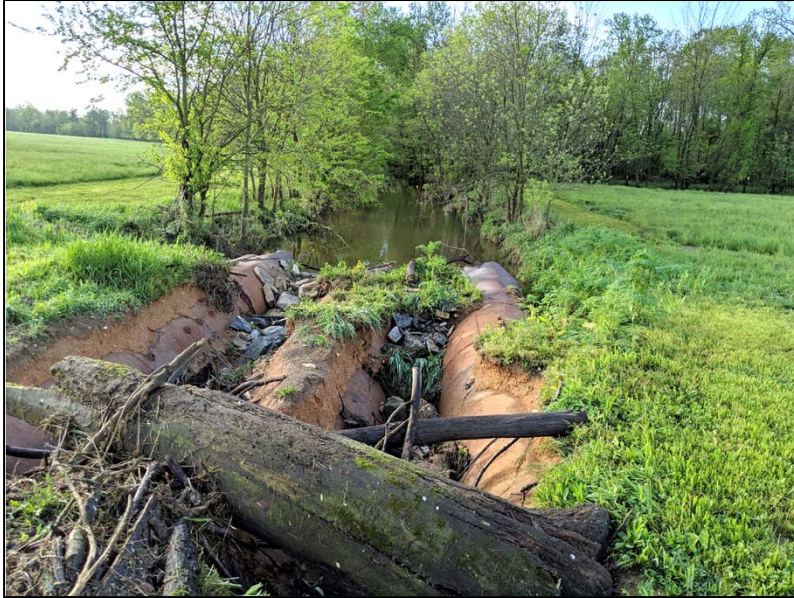
Photo 2 (5/6/2019) Viewing upstream section of failing culverts in Plum Creek and downstream limits of project.
