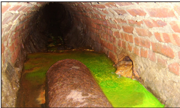
Green dye is used to trace the piping structure as water flows downstream. Photo by Don Ruhl
