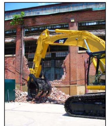
Crews remove one of buildings in Area 1 as part of the clean-up work.
