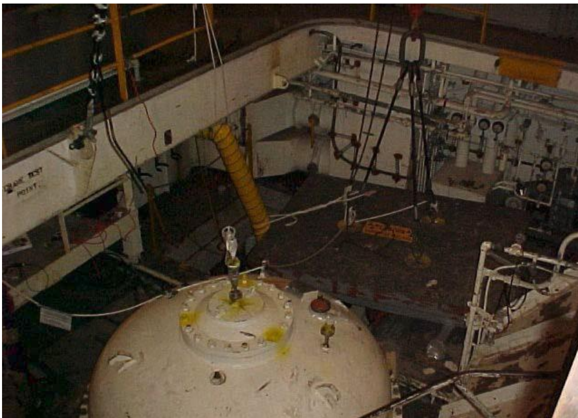
Figure 24. Refueling Room showing Spent Fuel Tank Lid and Access Plug (Honerlah and Hearty 2002).
