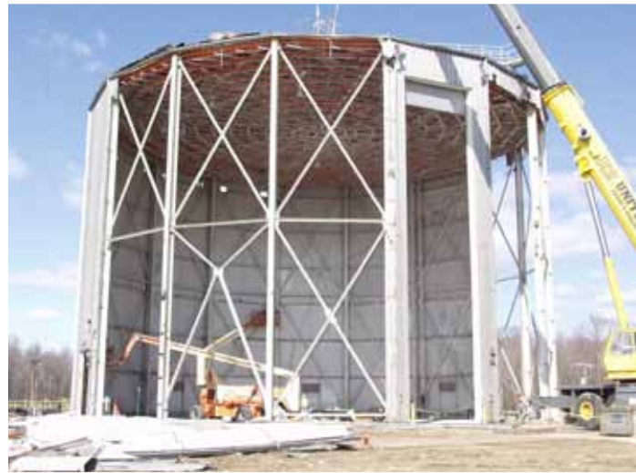
Crews conduct dismantlement of the Army Pulse Radiation Facility at Aberdeen Proving Ground, MD.
