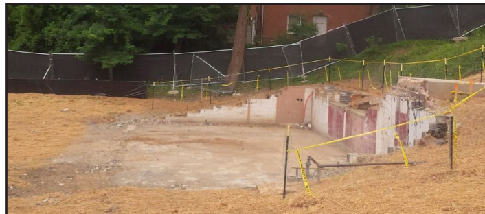
Foundation slab of American University's former Public Safety Building. Army Corps crews will remove the slab this summer and remove potential contamination below it that would have been associated with a nearby disposal pit that has already been cleaned.
