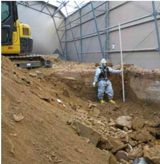
The team removed retaining walls, basement foundation walls, and the walkways in the front yard area of the property.
