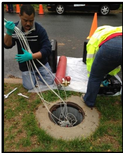
Multi-port Well Sampling on Glenbrook Road
