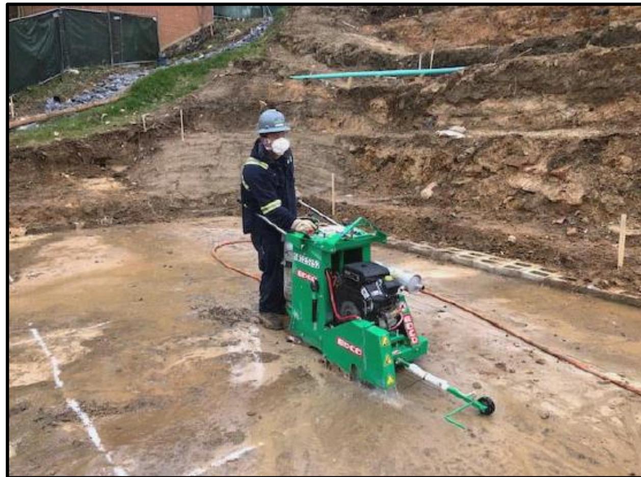
The crew using a walk-behind saw to cut the PSB foundation slab into sections. This saw distributes water to minimize the concrete dust.
