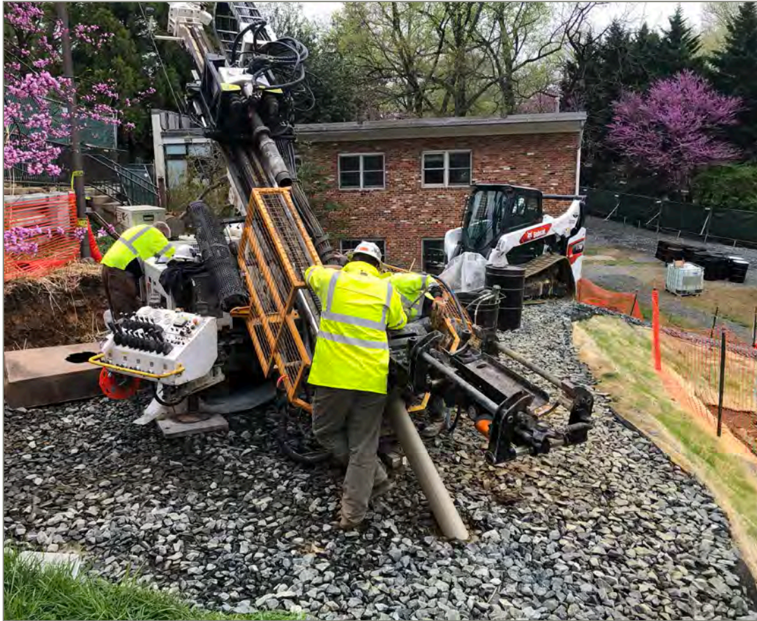
Rotosonic borehole RS-03 on drilling platform at the top of the PSB slope north of the foundation.
