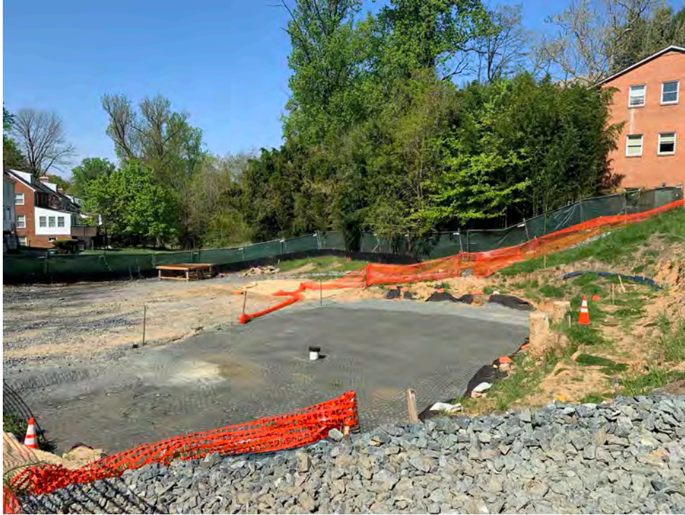
PSB Demobilized – Photo overlooking the site from the Rotosonic Drilling platform north of the PSB foundation excavation.
