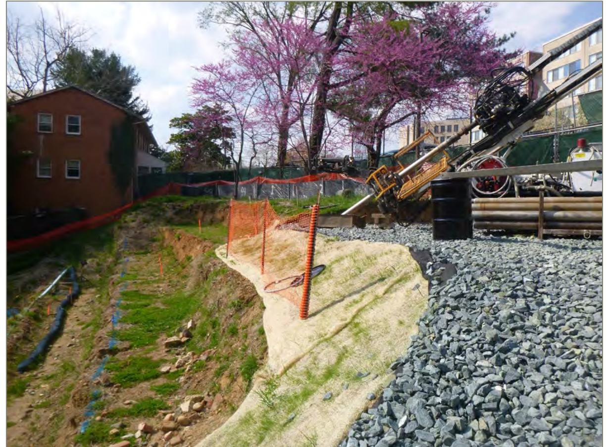
Rotosonic Rig advancing 4-inch diameter soil core barrel & 6-inch casing to collect continuous soil cores for AUES screening.
