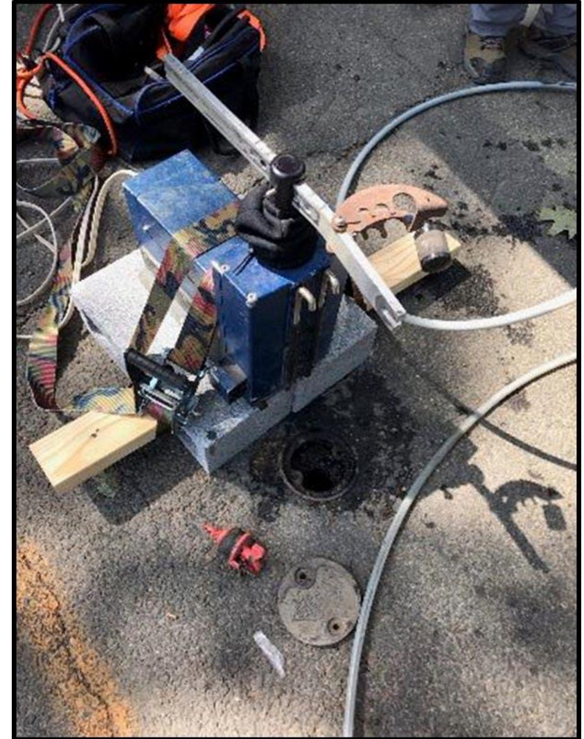
Groundwater sampling well
