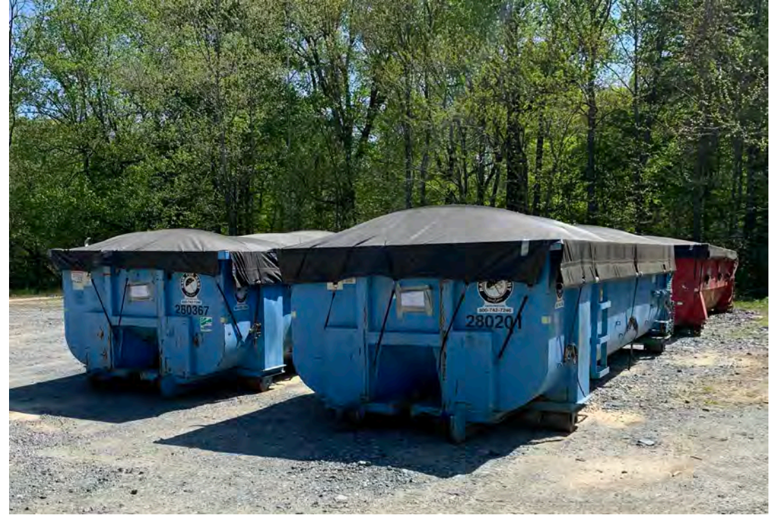
Waste Disposal – Last four excavated soil roll-offs waiting for disposal transport to King & Queen Landfill.
