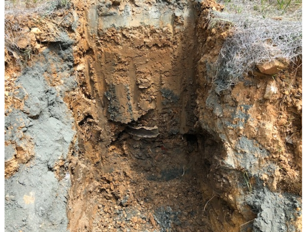
North Wall Grid D3 – Test pit into the North Sidewall – chasing the dark AUES debris layer @ 6 feet from slab.
