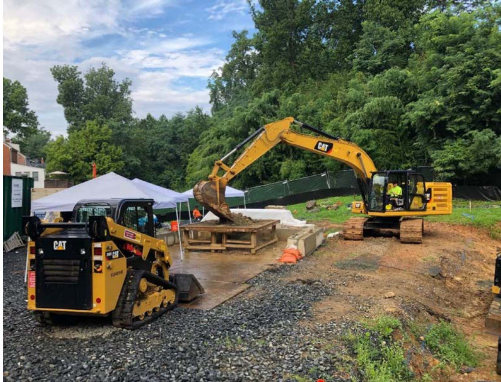
PSB Operations – Excavator dumping soil on the sorting table for the UXO Techs to screen for MEC/AUES items.
