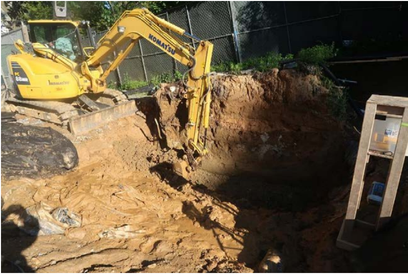
Excavation of the remaining portion of the north wall of Grid -10,-90 on June 7th
