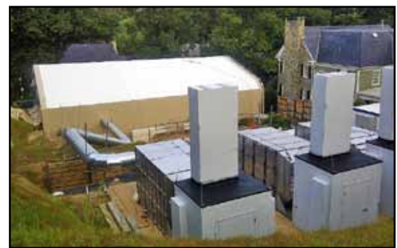
CAFS (foreground) installed with noise abatement at each unit, and the finished ECS (background).
